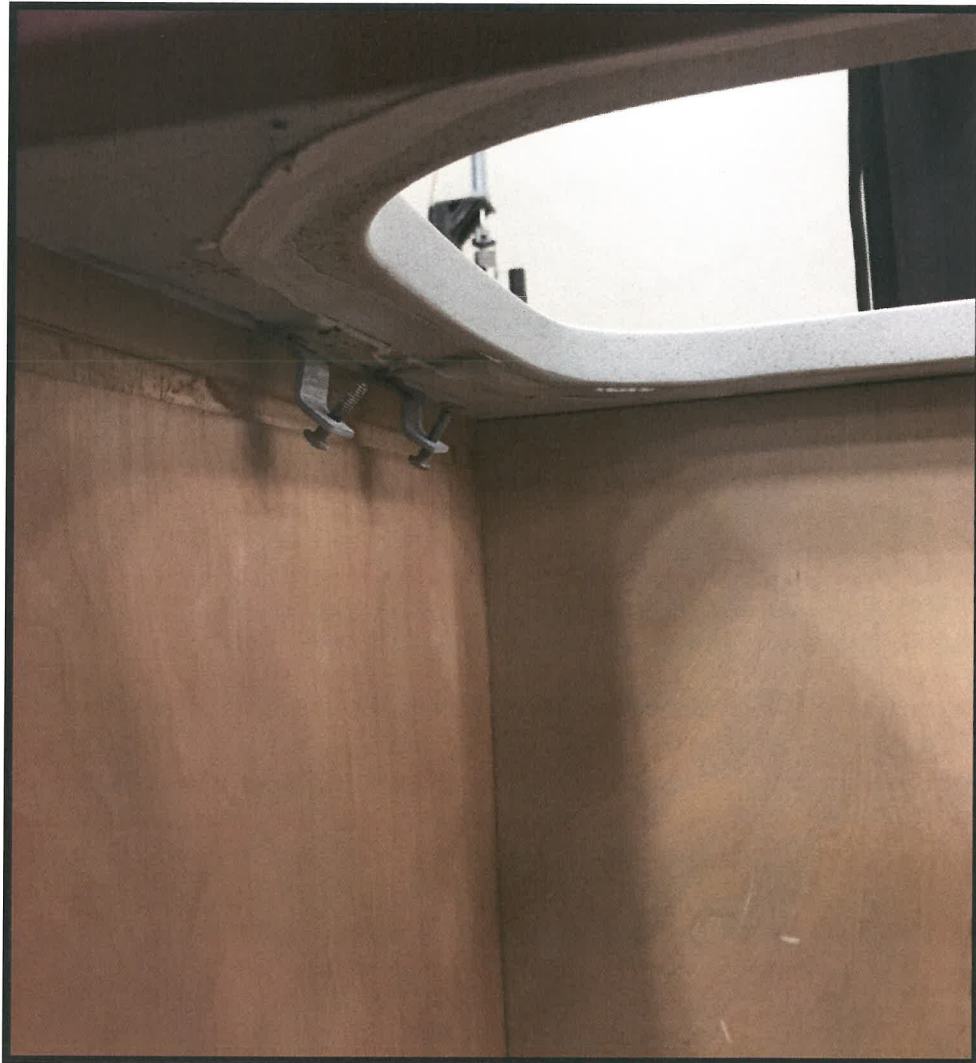
Figure 3: GoClips after failure
